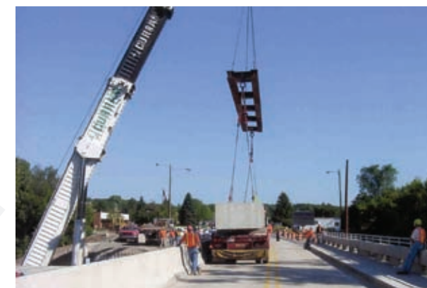
The Bridge Street Bridge project team earned the Precast/Prestressed Concrete Institute's prestigious Harry H. Edwards Industry Advancement Award. The engineering design and research team also was awarded the Eminent Conceptor Award – the highest award for engineering excellence for outstanding achievement for an engineering or surveying project – from the American Consulting Engineers Council of Michigan and the Michigan Society of Professional Engineers.
