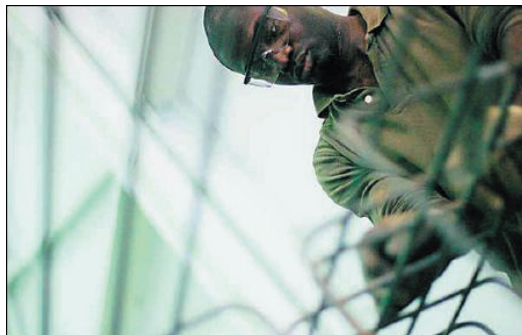
Joseph Hanson, 26, of Southfield works with other graduate students to build carbon-fiber cages for box-beam bridge supports at Lawrence Technological University.
