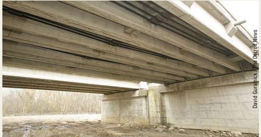
One span of the Bridge Street Bridge uses concrete and carbon fiber technology, which should give it a longer life span than bridges that have steel.
