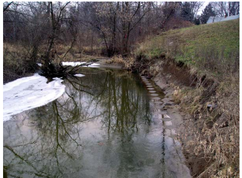
The eroded bank with the exposed 85 feet of interceptor sanitary sewer before the project (Dec 2006, Picture—R. Alsaigh)
