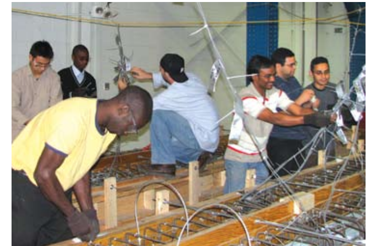
Before concrete is poured into forms for bridge beams to be tested at CIMR, Lawrence Tech students must check the tags on the sensors used to record load measurements. Pictured are (L-R) Joseph Hanson, Cheng-lin Wu, Delali Noamesi, project manager Tony Magnan, Prasadu Penjendra, Mheb Labib and Eslam Soliman.
