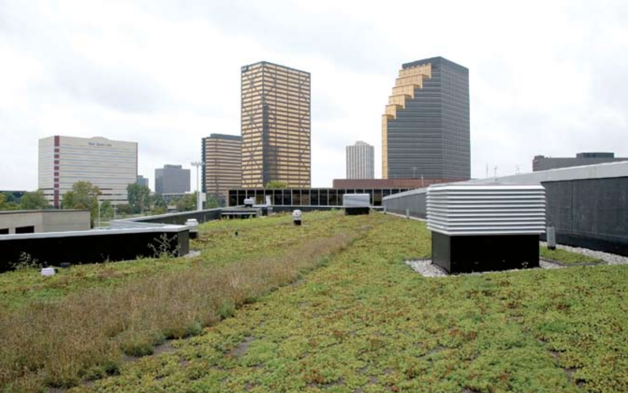
The 10,000-square-foot living “green” roof on Lawrence Tech’s Taubman Student Services Center consists of layers of insulation, roof membrane, drainage fabric, and a granular soil composition that supports nine different species of sedum. About nine inches thick, the roof offers more effective insulation than traditional roofs and expands and contracts with seasonal changes
