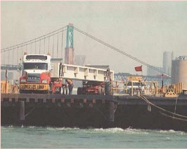
Test girder being barged across the Detroit River. Ambassador Bridge is in the background.
