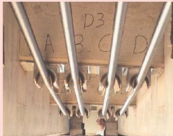
Underside view of test girder showing externally draped carbon fiber reinforced polymer (CFRP) tendons.
